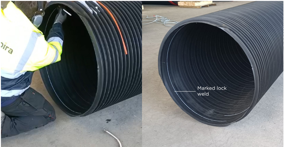
Figure 7 Picture of the lock weld being marked on the inside of the pipe (left) completed line in white (right)
